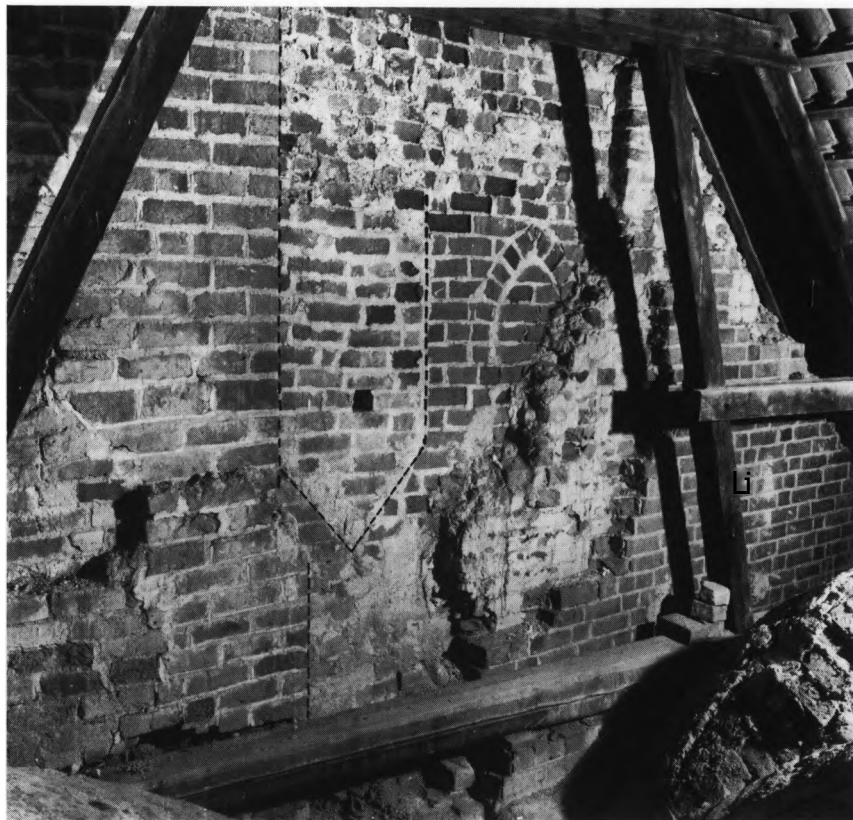
Fig. 9. Indersiden af nordre sideskibs vestre taggavl, set fra kirkeens loftsrums (s. 1248, jfr. fig. 3b og 8). HJ fot. 1984. - Inner face of the west gable of the north side aisle seen from the church loft (cf. fig. 3b and fig. 8). The junction between the gable and the then church's flanking wall to the north with cornice of stepped brick courses, as well as the bricked up opening for the valley between the two intersecting planes of roof are indicated by dotted lines.
